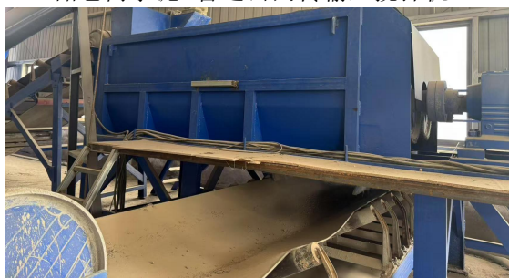
拌合楼全密闭
